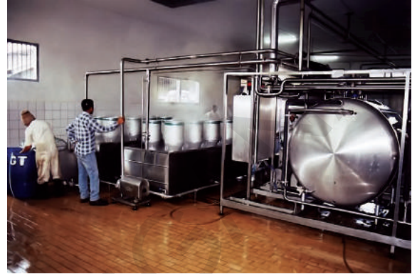
Fig-7 Chilling center
