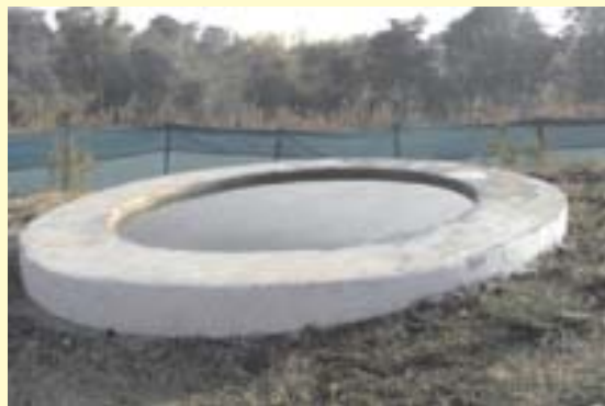
Water storage tank in nursery
