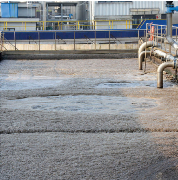
Sludge treatment and disposal
